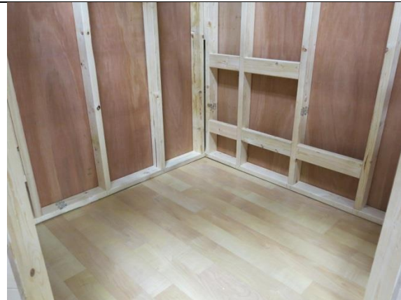
Photo 01. Notice location of bench support blocking.
